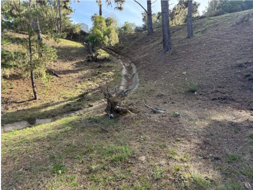
Photo 11. Representative view of concrete swales constructed on the site to direct stormwater runoff from the residential area along Skye Street down to lower bench area and storm drain pipe.
