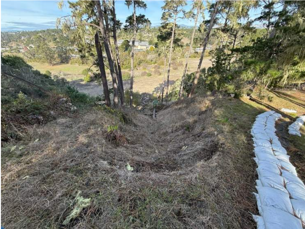
Photo 5. Northerly view of the eroded gully below the old road that is becoming revegetated by a mix of non-native and native plants.
