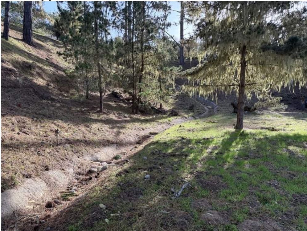
Photo 12. Additional view of concrete swales that direct stormwater from the upper slope to an existing storm drain pipe.
