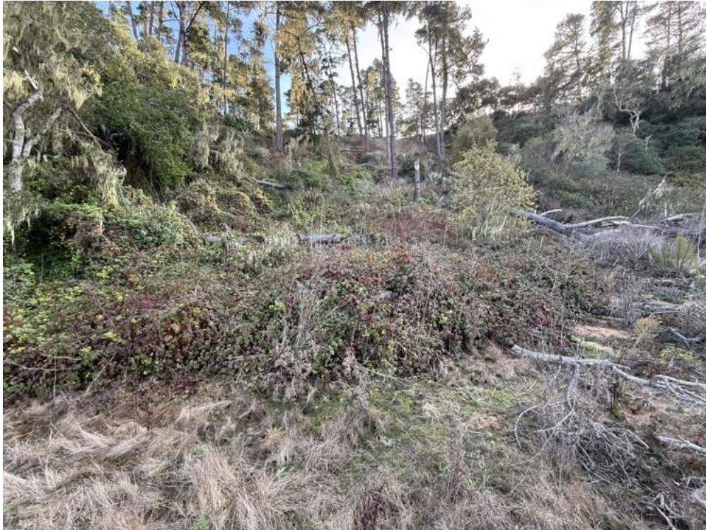
Photo 15. View of the lower slope showing dense vegetation with scattered Monterey pine and coast live oak trees. The storm drain pipe has been overgrown with understory plants.
