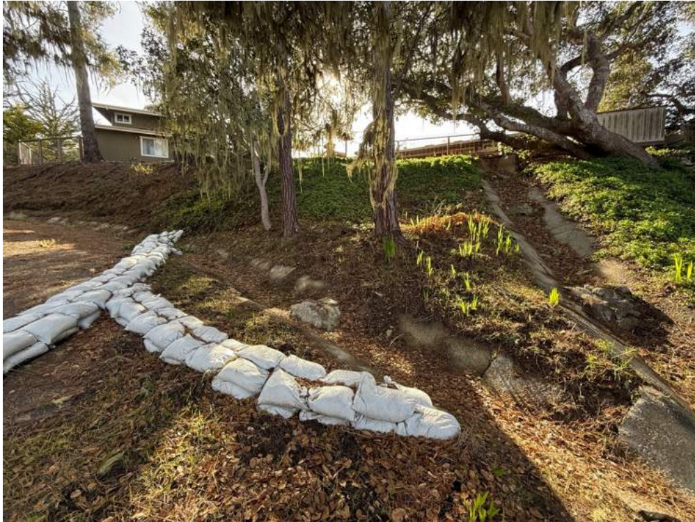
Photo 3. The concrete-lined swales direct surface runoff down the lower slope seen in the right bottom corner to a culvert and storm drain pipe on the steep slope.
