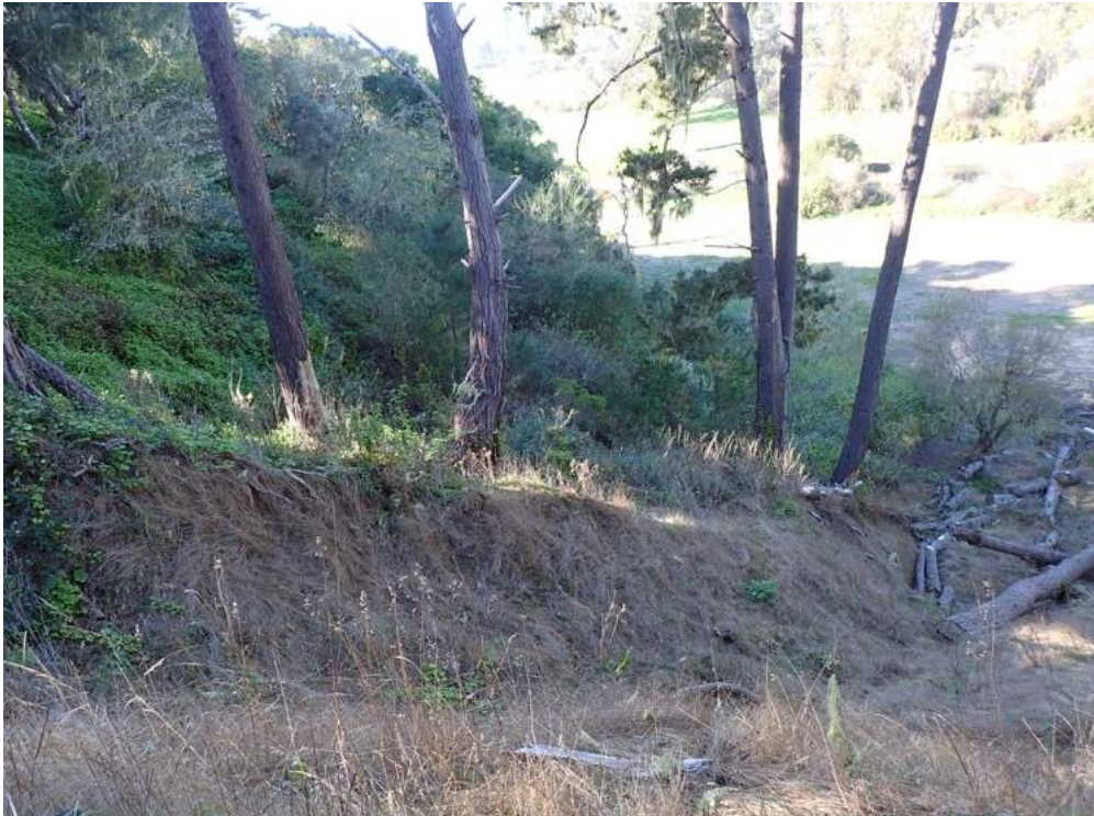
Photo 6. Another view of the erosion area showing existing vegetation. Remnant tree trunks that were in the erosion area are visible near the toe of slope on the far right.
