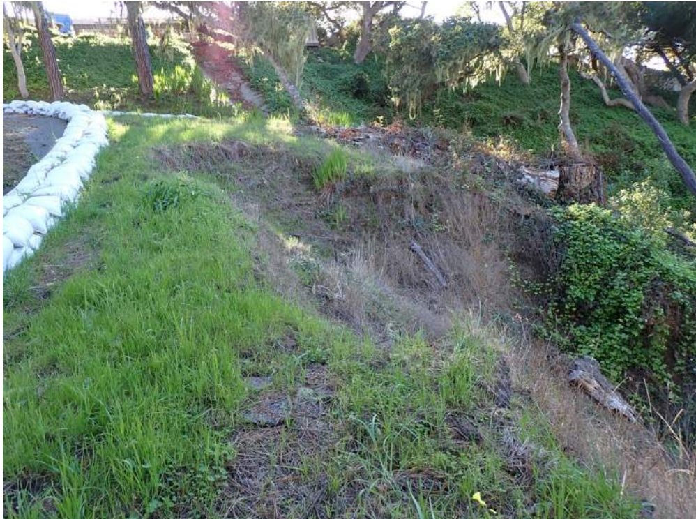
Photo 4. During winter 2022-2023, surface runoff down the road bypassed the drainage structures and eroded the hillside below the road.
